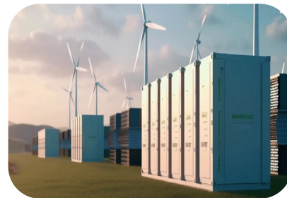
Large stationary storage systems
